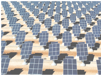
Solar photovoltaic array
